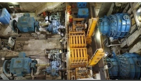
8MW Hydro Plant
